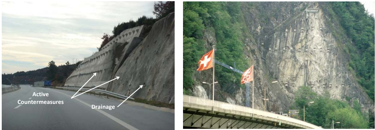
Figure 15 : Examples of slope stabilisation measures from Switzerland.
