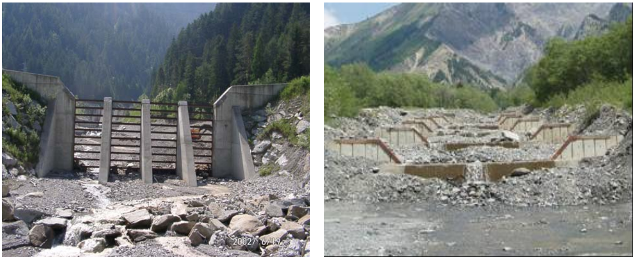
Figure 14 : Examples of physical protection measures against debris flows from Austria (left) and France (right).
