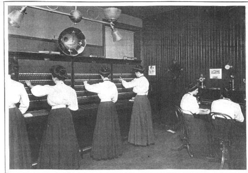
Left-Hand Side of "Music Room" in the Telephone Exchange at Wilmington, Delaware.
